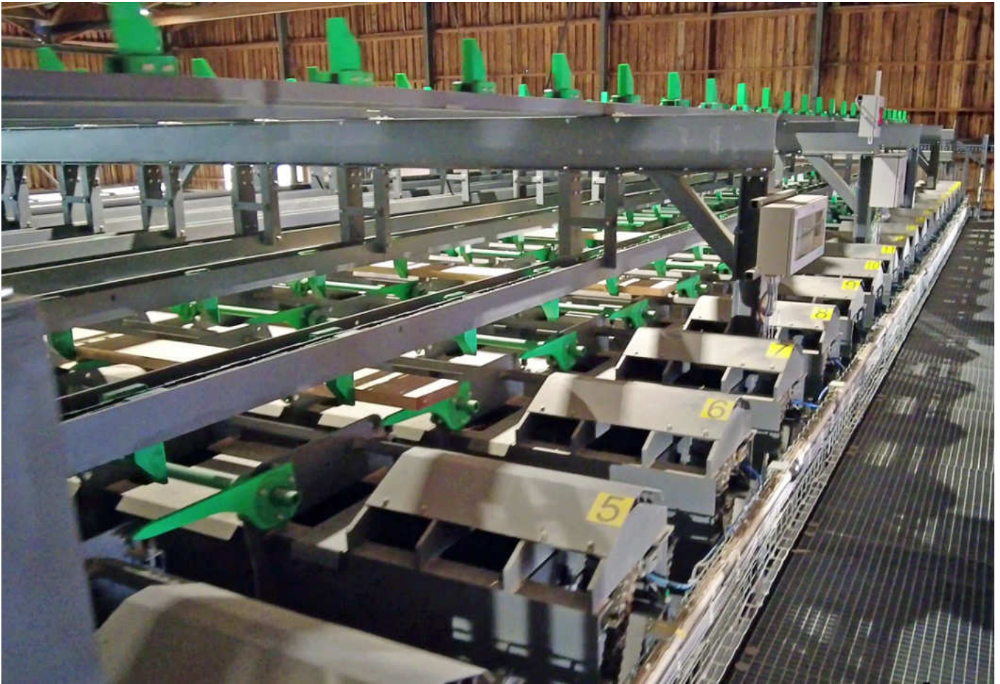
The 22 boxes in the new sorting plant prevent bottlenecks (Pic by Kallfass).
